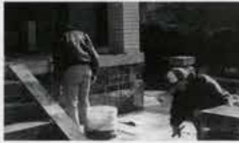
Masonry workers restoring the Chinese Temple at Naumkeag. Courtesy The Trustees of Reservations.
